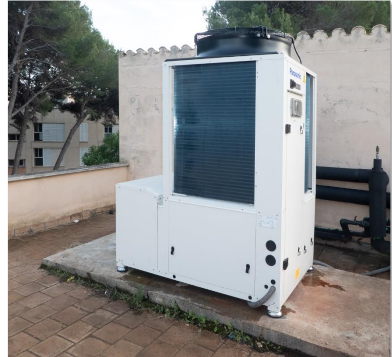
40 kW unit with 100 l buffer tank
