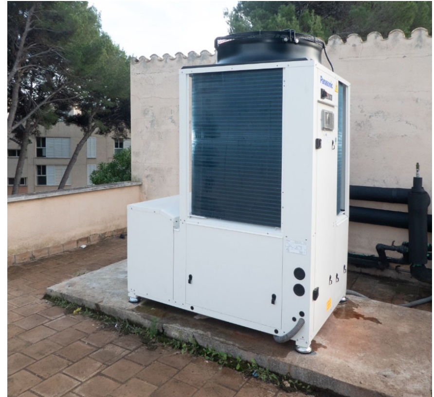
40 kW unit with 100 l buffer tank
